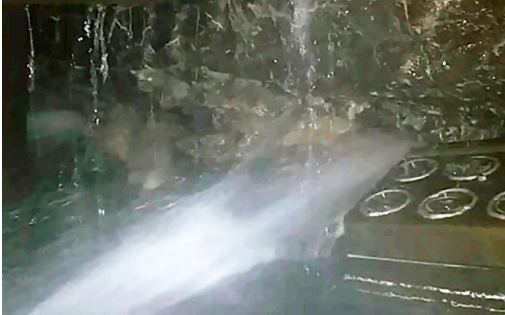
Figure 17. Pressurized groundwater entering at the tunnel face in the R3 Metro Line tunnel in Jinan, China (Kang et al. 2021).
