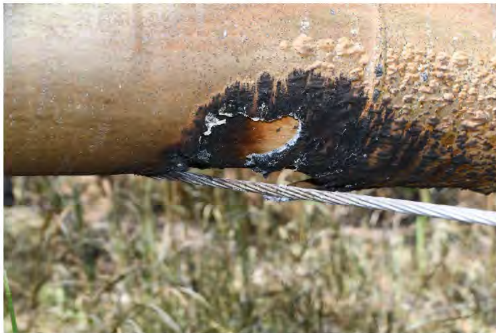
Arcing on conductors (JMD_4254)
