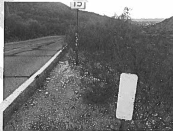
Object markers to be replaced.
