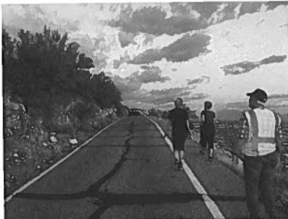
Guard rail segments, better object markers, and/or delineators recommended to better guide vehicles in the narrow road.
